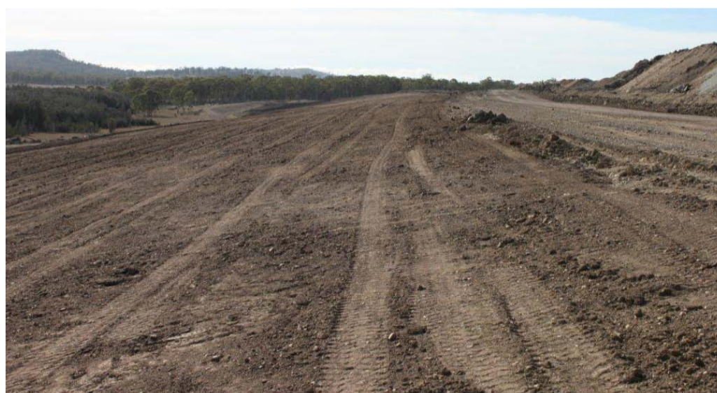
Bulk shaping undertaken on Northern face of Noise bund near Wybong Road.
